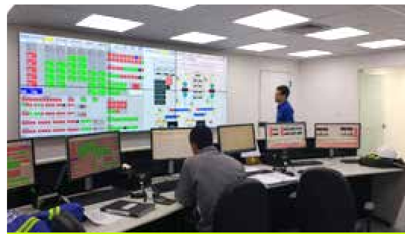
Figure 1. Operational Control Center of the Copersucar Sugar Terminal (TAC)
